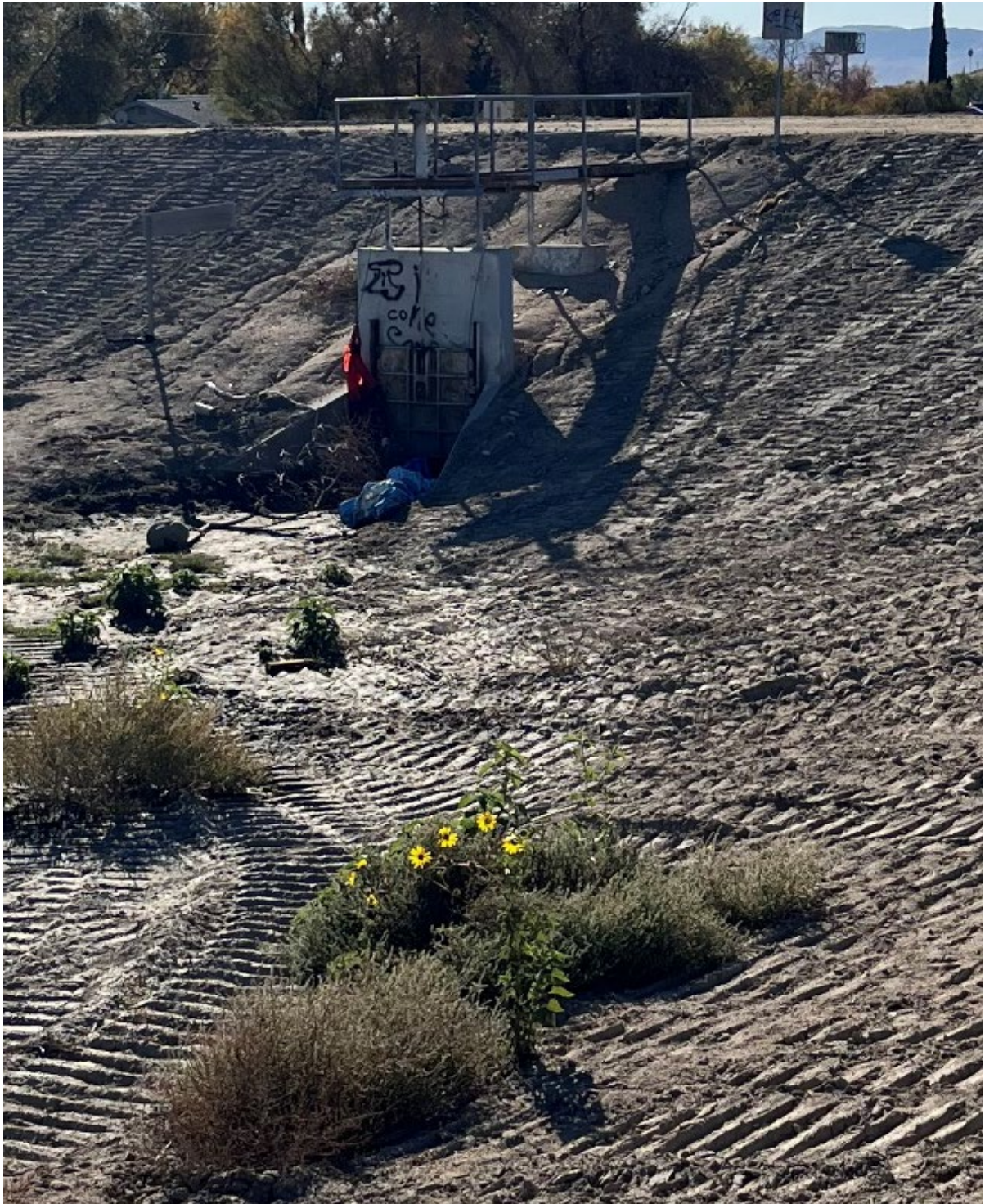
Figure T- Lynwood Basin No. 1: 48-inch diameter slidegate over outlet – observed in full open position Nov. 20, 2024
