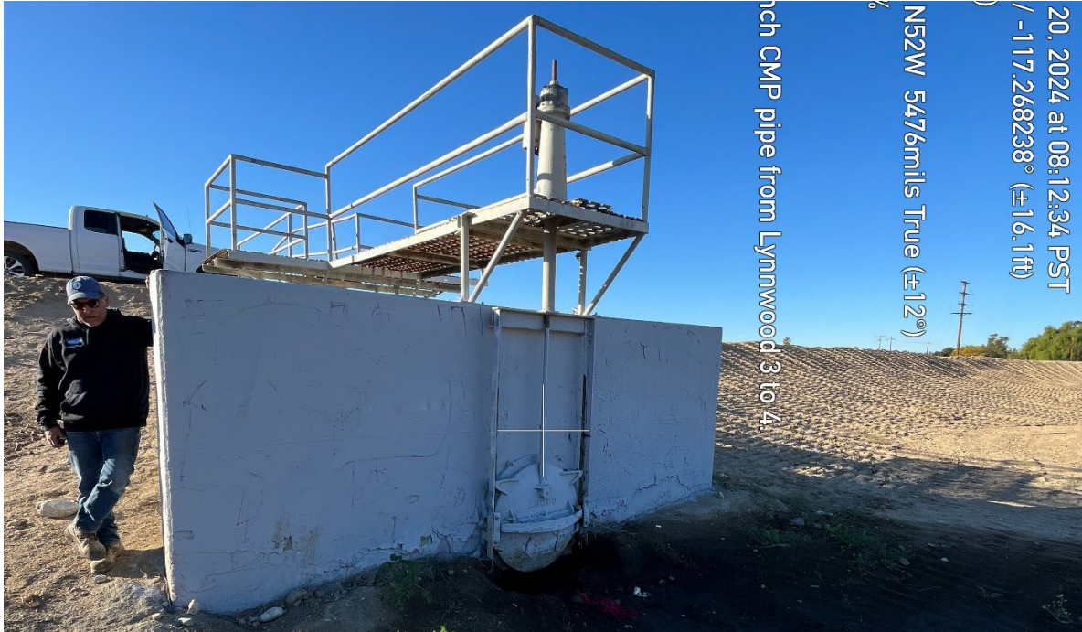
Figure U- Slidegate over outflow in forefront of drop-inlet structure typical for Lynwood Basin Nos. 2 and 3
