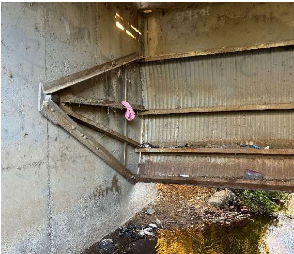
Figure M East Bay Radial Gate Frozen Open at 1.8 feet - INOPERABLE
