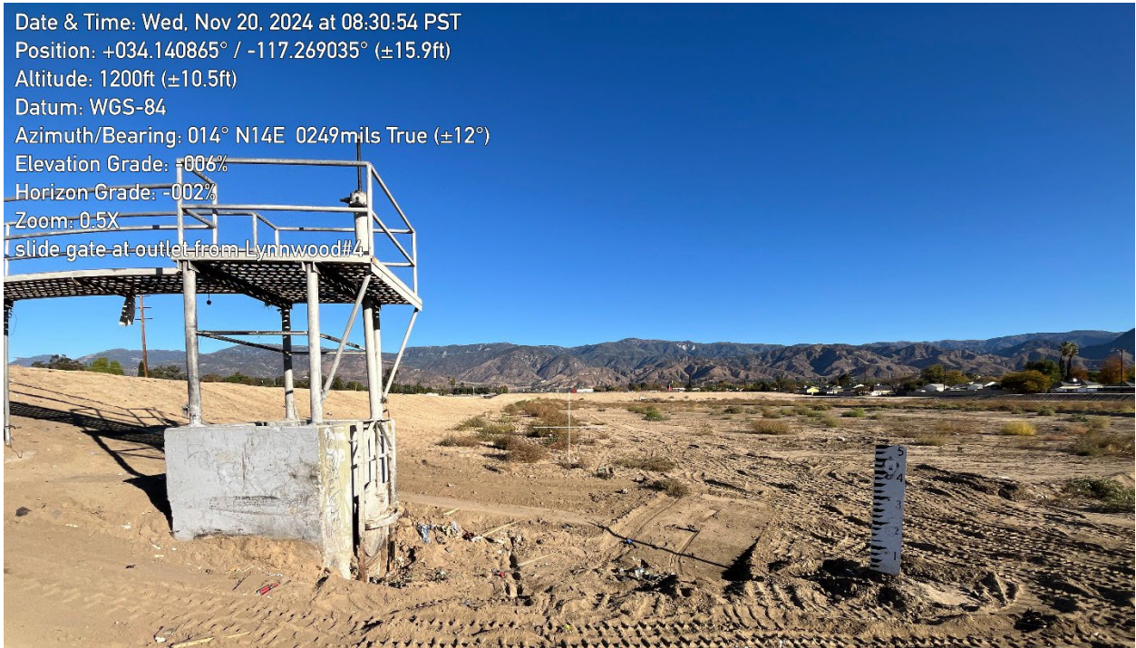
Figure X - Lynwood Basin No. 4 36-inch diameter Slidegate over outlet pipe - Observed open on Nov. 20,2024
