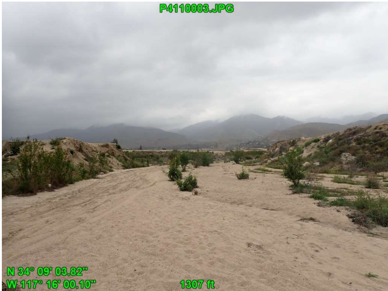
Figure N Breached Internal Berm in TCRB Existing Conditions
