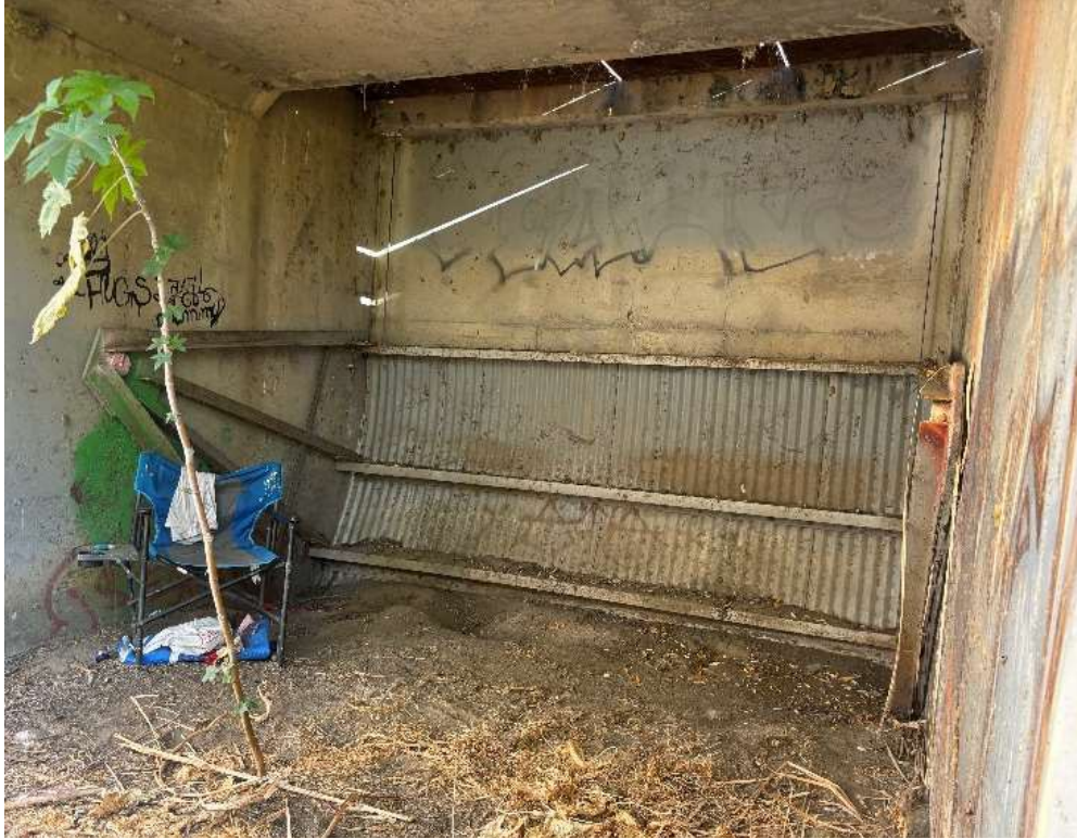
Figure L West Bay and Radial Gate at Heading 1C - INOPERABLE
