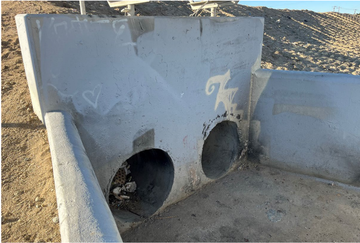
Figure V- Sidewall of drop inlet to dual-pipe outflow culvert at Basin Nos. 2 & 3 (picture where man was standing)
