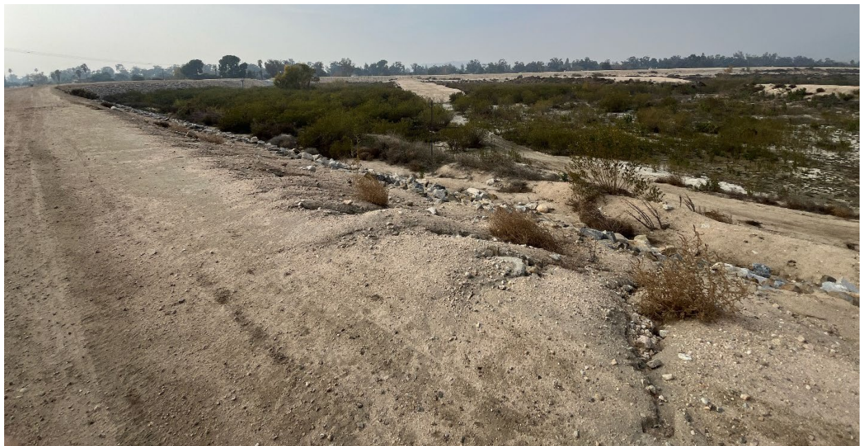
Figure O Southern Flood Levee at TCRB Looking East - RC Channel Entry and Drain Gate Visible in Background
