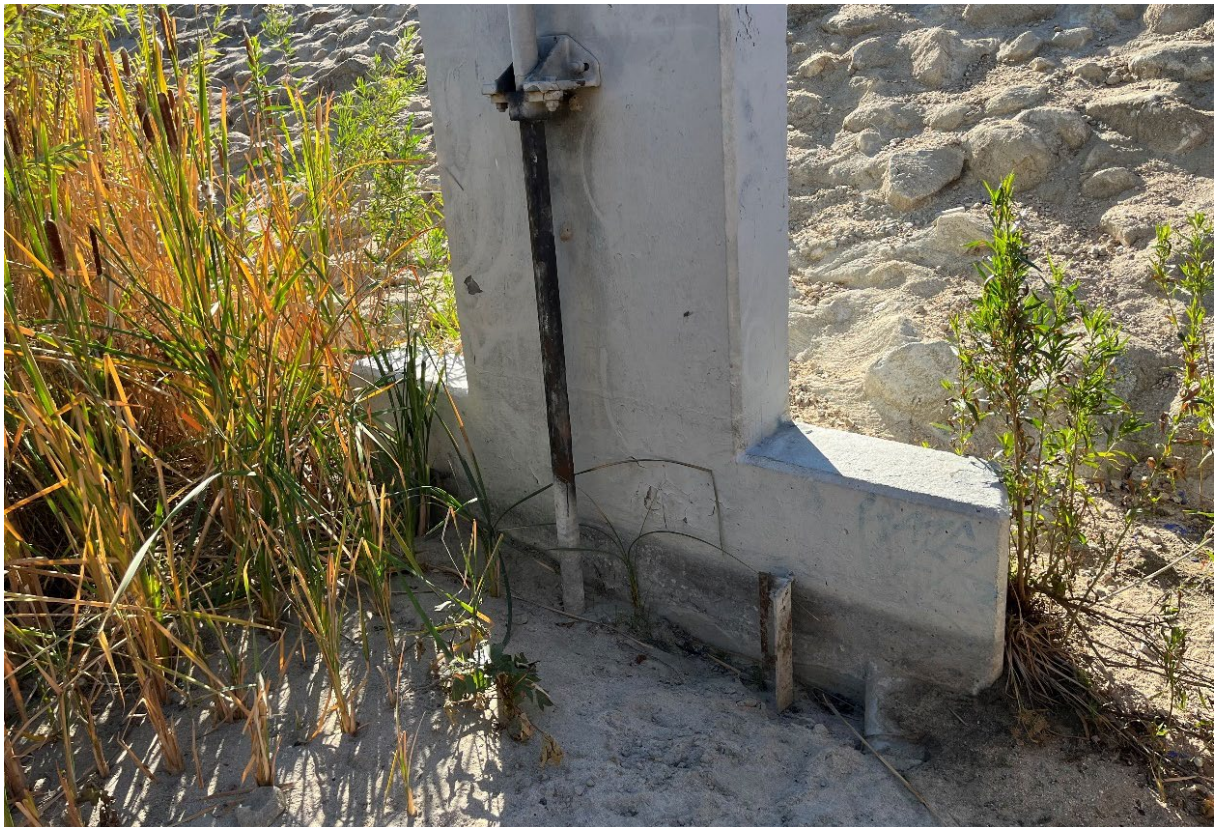
Figure R - View of TCRB Drain Gate buried by deposits of sand
