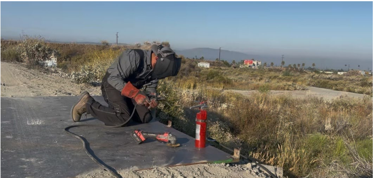
Tommy Purvis welds steel plates installed to replace grates on a District road on July 27
