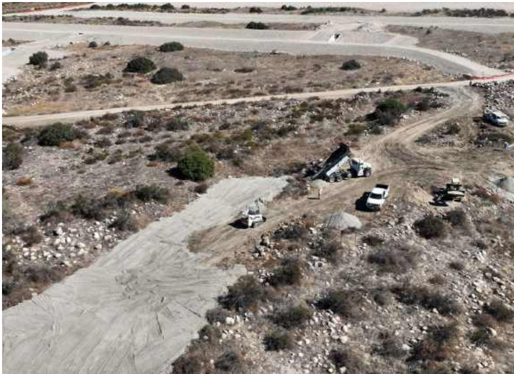
Work to decrease fire risk implemented by the BLM Fuel Management grant on October 22
