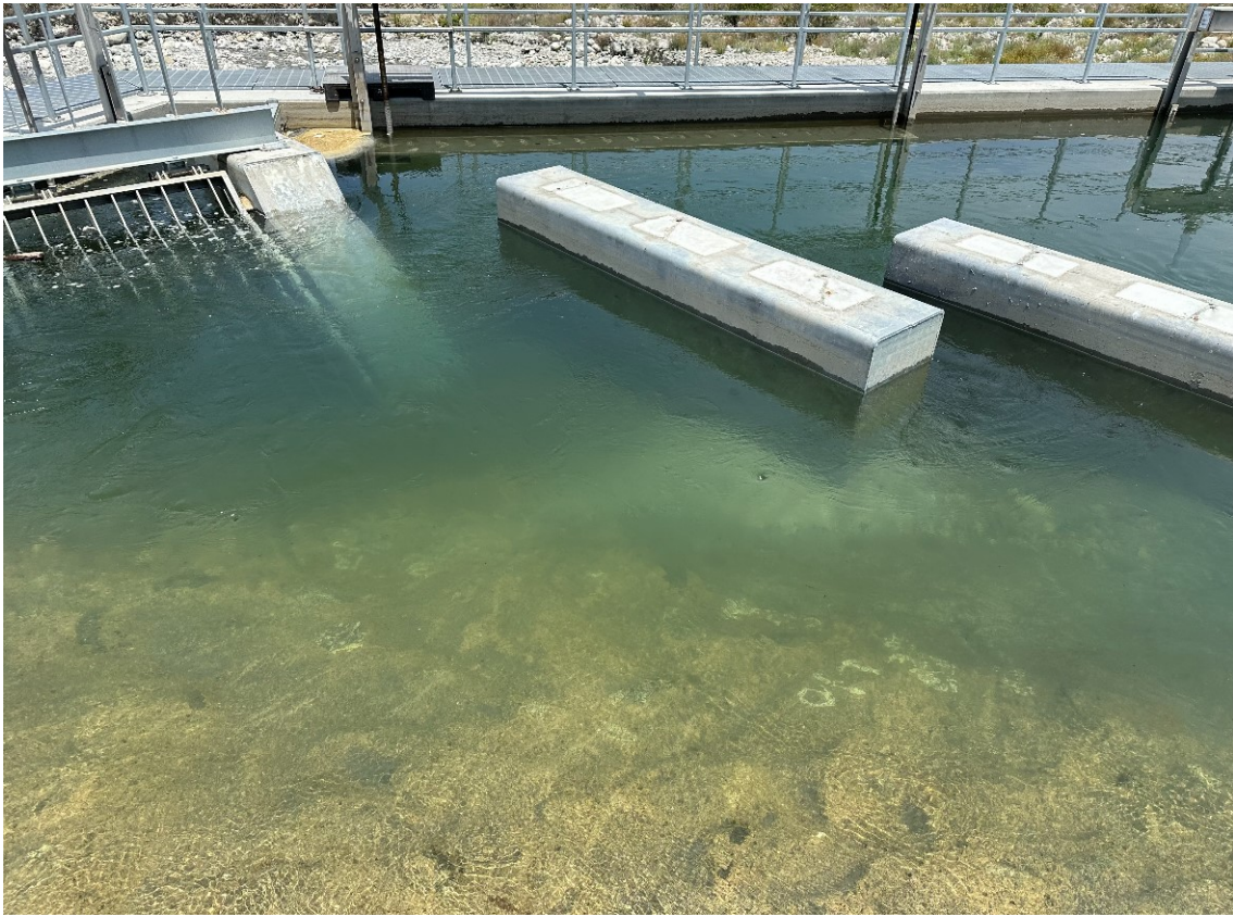
Clean, clear snowmelt being diverted through the new Mill Creek Diversion for recharge
