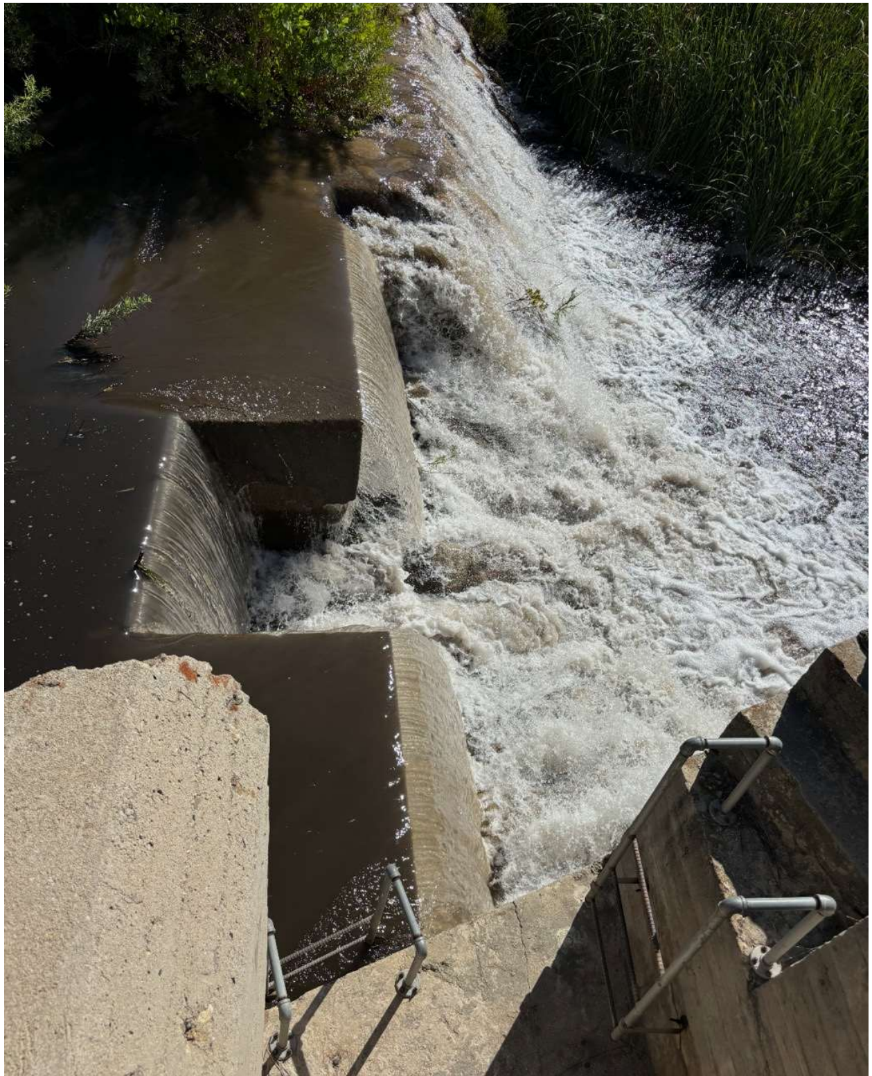
Water with a high post-fire sediment load being routed to the sedimentation basins for cleaning during the Line Fire on September 23
