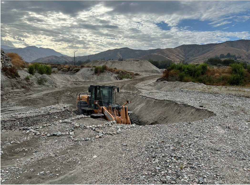
Tommy Purvis operating leased equipment to remove sediment from Mill Creek recharge basin.
