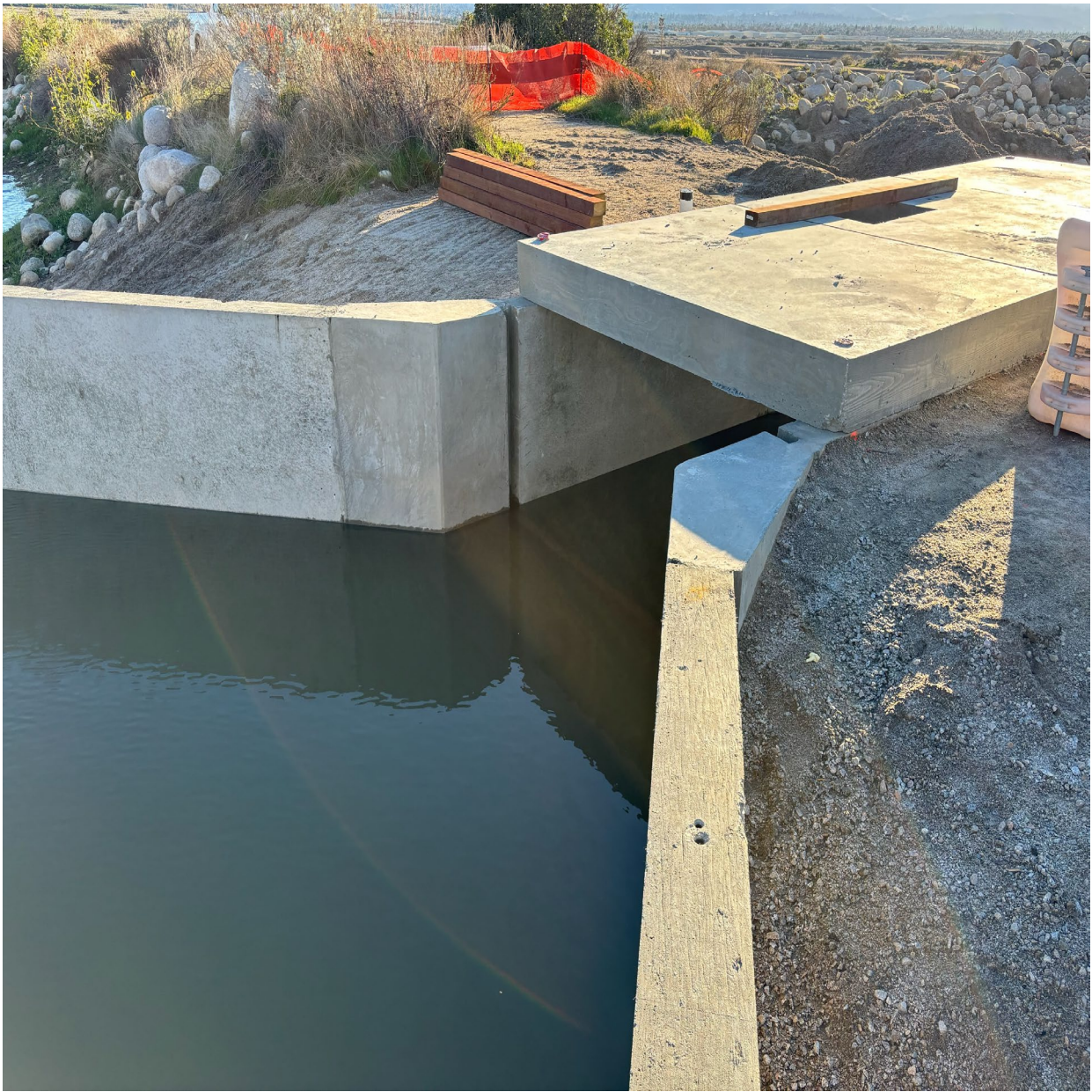
Water building up to spill into the first completed Enhanced Recharge basin
